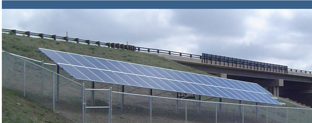
Solar site on the NWP Right-of-Way slope.
